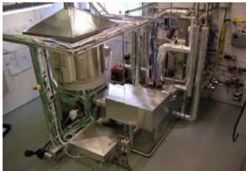
SOFC 1 - 5 kW test system NG, 2004, > 3500 h in operation
