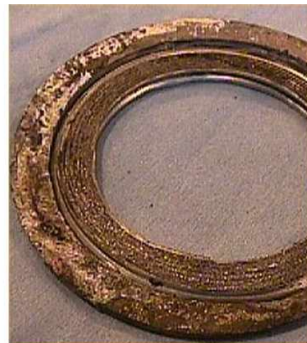
Crevice corrosion on the face of a flange caused by absorbent gasket, also known as gasket corrosion
